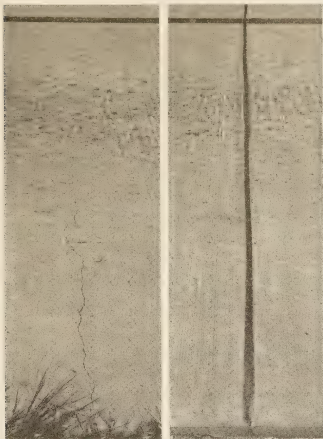
FIGURE 21.—LEFT, CRACK THAT HAS OCCURRED AT A SUBMERGED WEAKENED-PLANE JOINT; RIGHT, WEAKENED-PLANE JOINT WITH SURFACE GROOVE.
